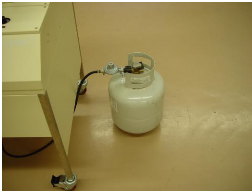
Liquid Propane (L.P.) Cylinder Fuel used to power boiler
